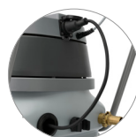
Plug powering discharging pump
